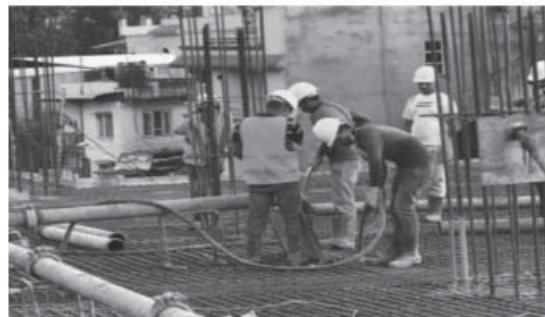
Figure 1 Hazards at Building Construction
